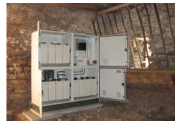
System-Voltage: 230 V AC | Photovoltaics: 540 Wp | Battery: 15 kWh | Inverter: 2300 W | with UPS | Batterie Charger: 0 – 55 A | Location: Valais - Switzerland
